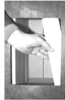
15. The long thin front brick can now be fitted in the remaining space at the front right of the firebox...
