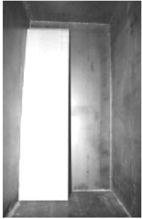
1. Fit the 2 back bricks by initially leaning them against the back of the firebox as shown to prevent them from falling forward.
